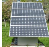
Solar Power Station
